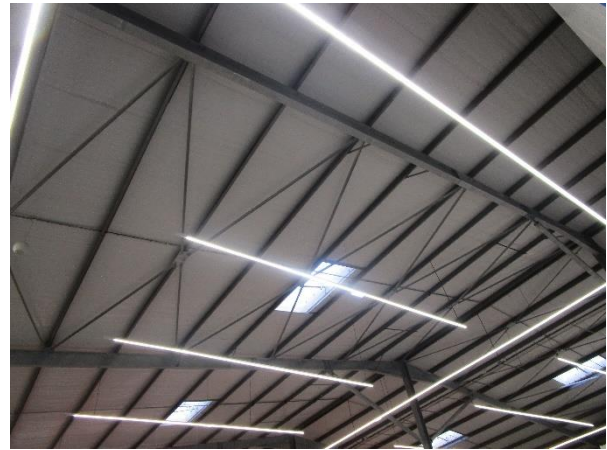
Photo 46 - Ruban LED de surface commerciale
